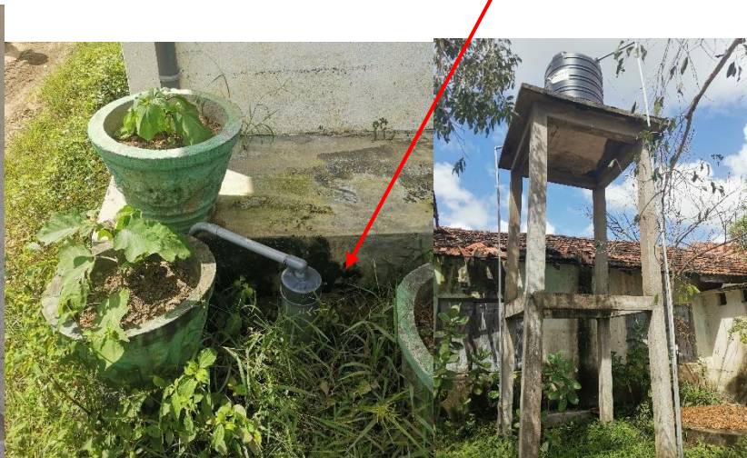
Drinking water facilities - Tube well & water tank
