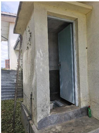
Toilet - Poor condition
